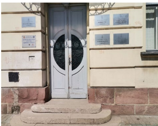
Photo 3: inaccessible main entrance, the basic court in Pirot
